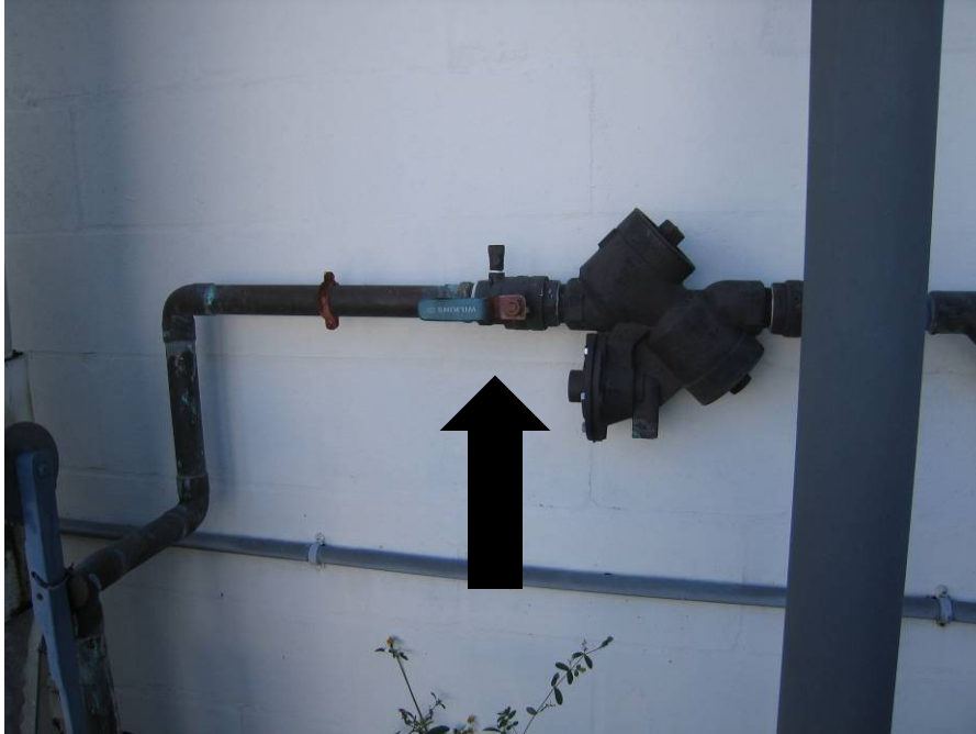
Chiller Yard - Water Isolation valve shown in the ON (open) position OFF (closed) - Position handle perpendicular to the water line
