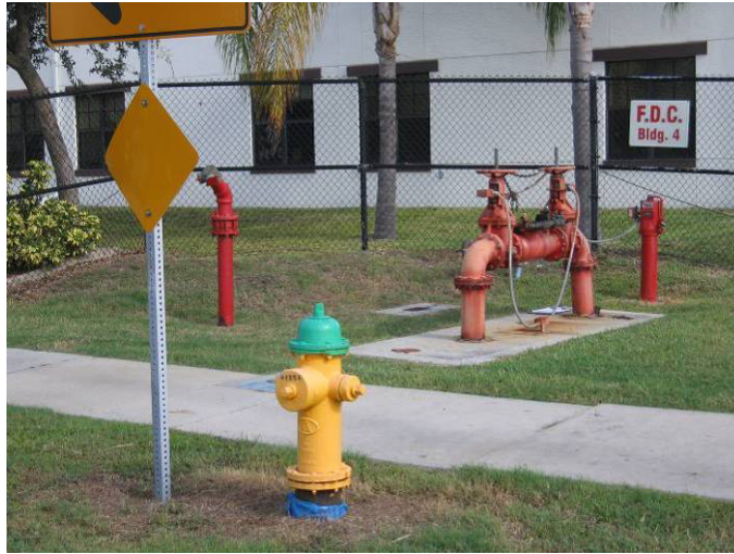
Fire Department Control Valves and Attach Stub up – Do Not Operate
