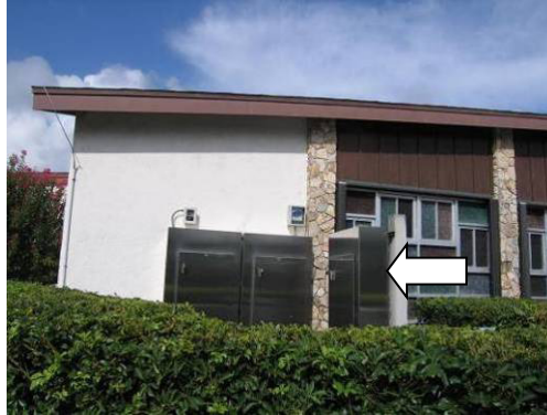
Power Breaker Boxes Sanctuary - South East Corner
