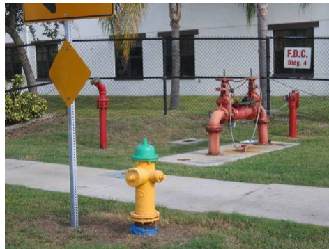
Fire Water Supply - Hatfield Street
